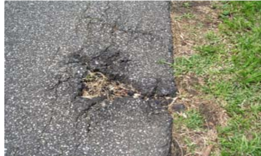
Damage to path – possibly by tree roots
