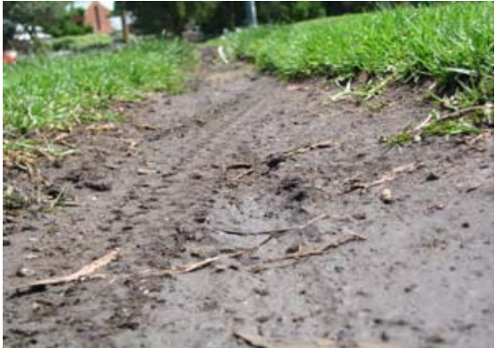
Shortcut – showing damage/erosion.
